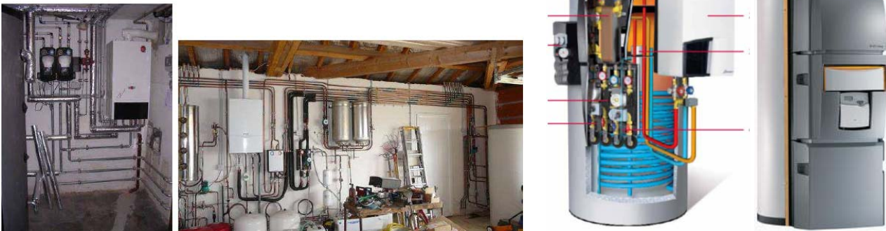
Fig 2. Examples of often existing bad hydraulic installations (left) and examples for compact solutions with minimized pipe length within the system (right) [4]
